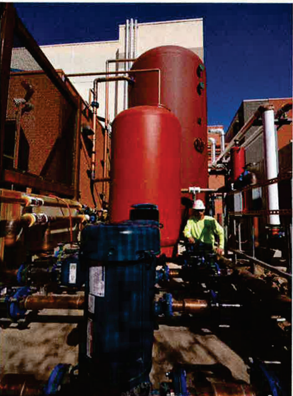
Top: W.J. Maloney Project Manager Travis Brock inspects a heat exchanger. Above: Pumps (blue), an expansion tank (smaller red tank) and a storage tank (larger red tank) are part of a system that yields year-round efficiencies.
